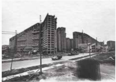
Construction of public housing flats in Potong Pasir estate in the mid to late 1980s.
